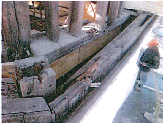
Figure 2 – Deteriorated Column and Beam Failure
