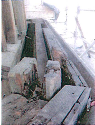
Figure 7 – Failed Column/Beam Connection
