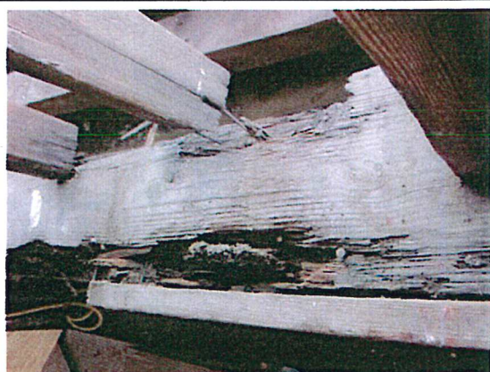
Figure 4 – Damaged Sill Exposed
