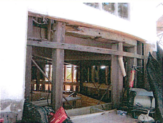
Figure 3 – Damaged Sill Beam
